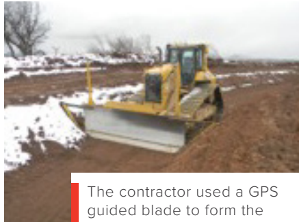
MegaDitch lined irrigation channel conveys much needed water to ranchers.
