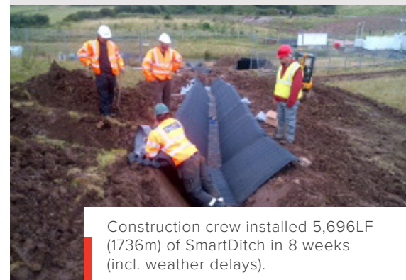
SmartDitch is already hard at work before the installation is even complete.
