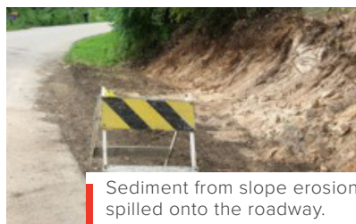
Drainage ditch was shallow, overgrown and has a large eroded section.
