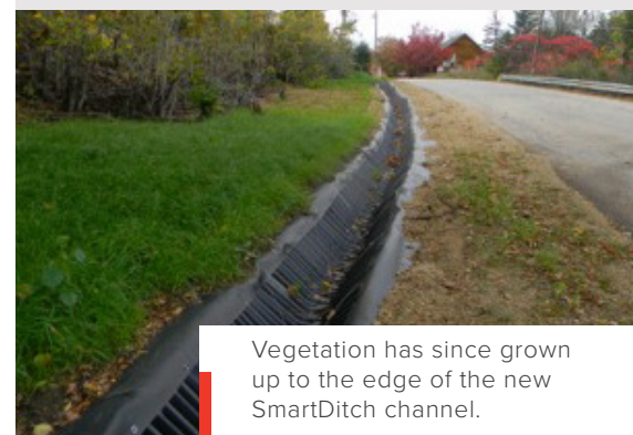
The town of La Valle's own maintenance crew installed the 12" depth SmartDitch channels.
