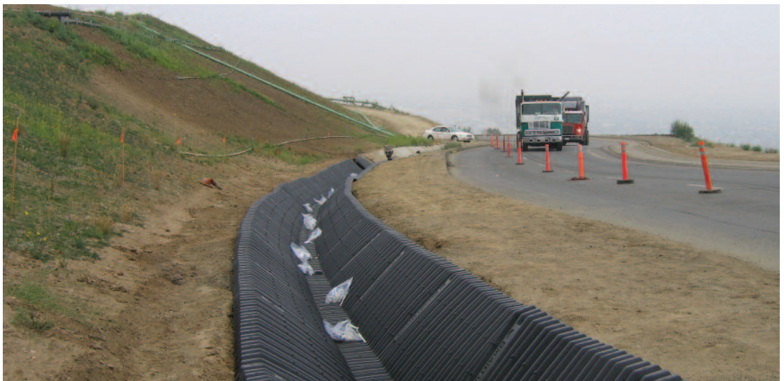
Initially, SmartDitch was installed in a channel at this Puente Hills Landfill site to temporarily control a conveyance ditch. However, considerable settlement over time made the use of concrete channels (originally specified) unusable and SmartDitch became the permanent solution.
