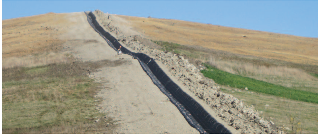
2,750 feet of 24" Trapezoidal SmartDitch Liner was used to control erosion and stabilize slopes at the Newton County, Indiana Landfill. SmartDitch's proven water flow control characteristics, low maintenance and ease of installation made it the best option for this project. The bulk of this installation took just 3 days and a crew of 5.
